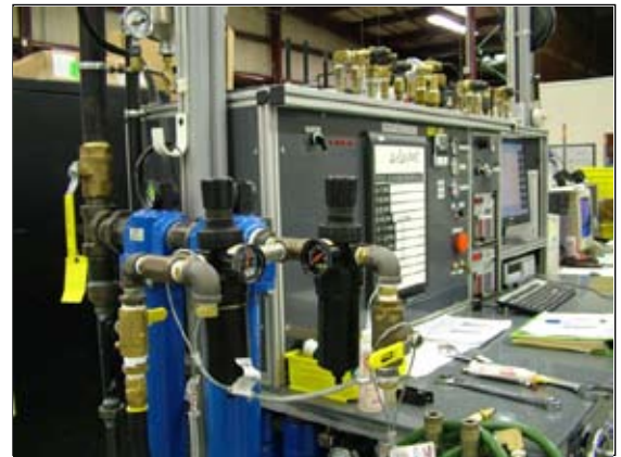
Critical test station serviced with Balston Filter Regulators and Large Prefilters
