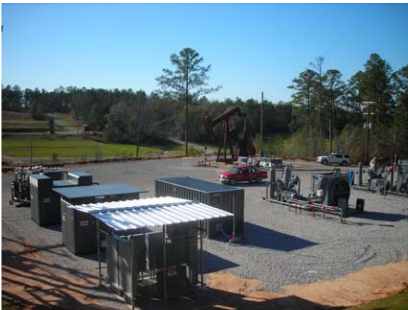
Feed air compressors (left), membrane container (center) and booster compressors (right) on customer's location
